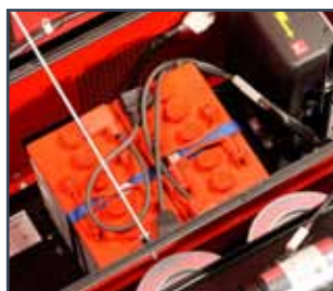
NO.4 BATTERIES 6V-240 AH (20h) - (E) 4 BATTERIEN 6V - 240AH (5h) 4 6V-240AH (5h) ACCU'S
